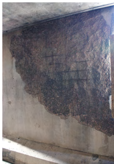
Spalling observed after a fire in a parking garage. Courtesy of Robert McNamee.
