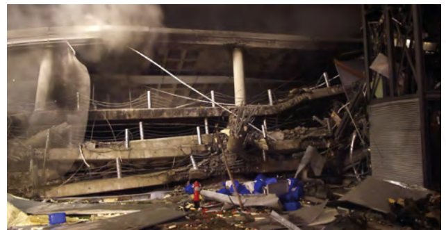
▲ Barajas Airport, Terminal T4 Parking Building - 30 th December, 2006. Courtesy of Alejandro Pérez Caldentey.
