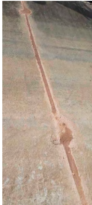
Filling of the joints between water channels covered with concrete slabs ©TC282-CCL
