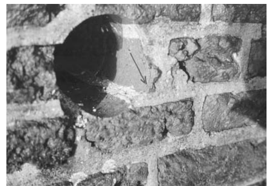
Fig. 3 - Start of damage visible in the hole left by the drilled core (see arrow for location): a layer of the brick begins to detach, the bedding mortar shows loss of cohesion.
