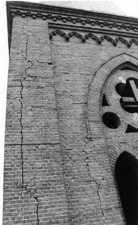
Fig. 1 - Wide (vertical and also horizontal) cracks, on the first sight looking like structural cracks, were found to be caused by swelling compounds in the inner part of the masonry.
