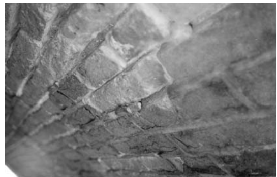
Fig. 2 - Damage in the passage(way) of a historical arch bridge: spalling of brick and pointing is pushed out.
