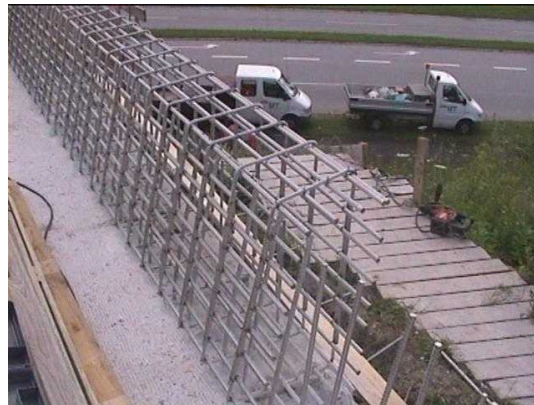
Figure 12: Danish Motorway. Selective use of stainless steel reinforcement for edge beams
