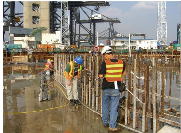
Figure 9: The outer layer of reinforcement of the Stonecutter Bridge is stainless steel. The remaining is ordinary black steel.
