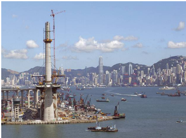
Figure 8: Stonecutter Bridge, Hong Kong. Design: COWI A/S in Joint Venture with Arup
