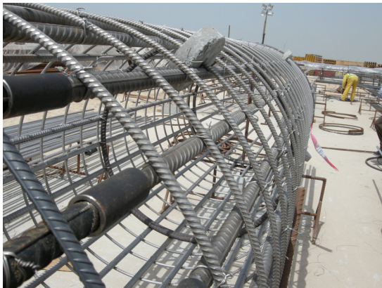
Figure 11: Mix of stainless steel and ordinary black steel at piles, AL Khail Road Interchange, Dubai
